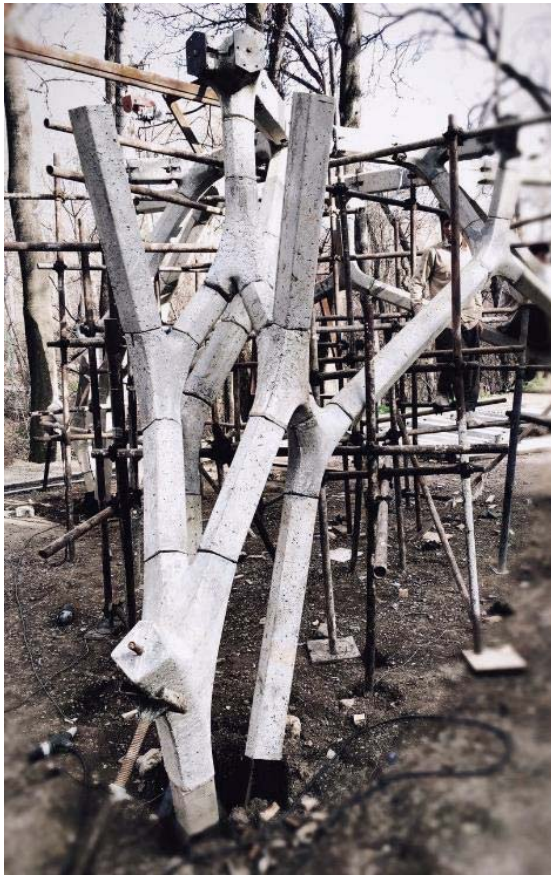
Figure 8: A photograph during the assembly process showing a compressive joint (bottom) and a tensile joint (top), dry connections between the compressive joints and members, and the conventional scaffolding system to support the unfinished structure.
